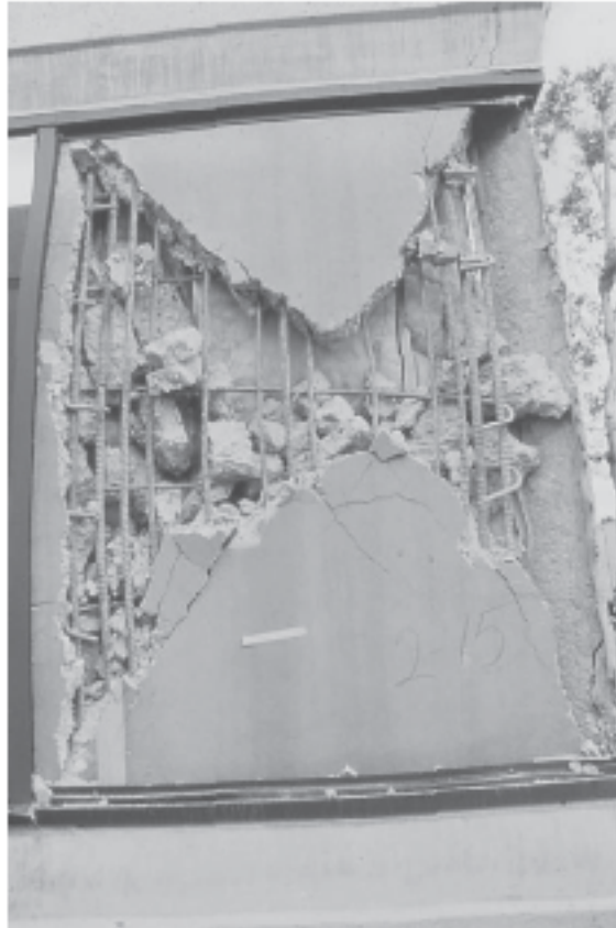
Photo 1.6 Overreinforced wall panel shear failure, Northridge earthquake, 1994. (Courtesy of Englekirk Partners, Inc.)
