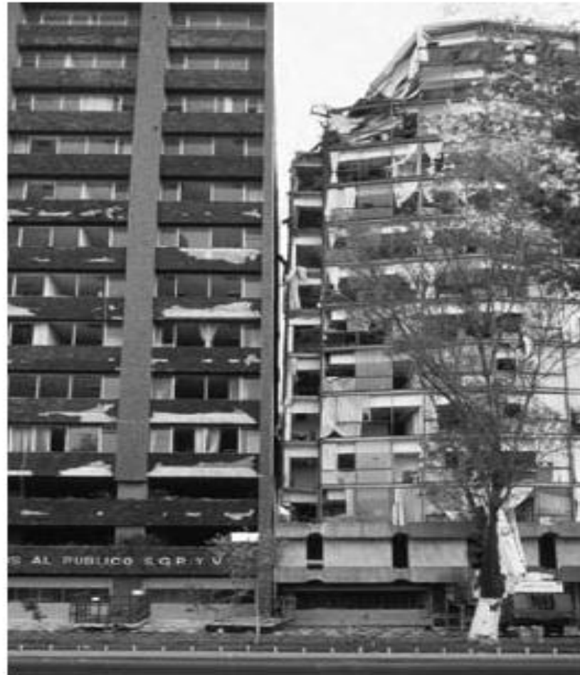
Pounding damage during the 1985 Mexico City earthquake. (Reproduced with permission from David C. Hopkins).
