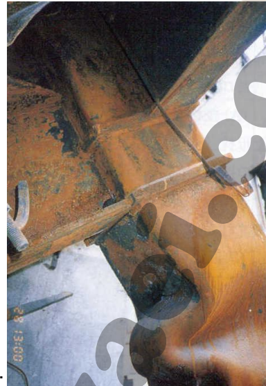
Local buckling of an HSS column....
