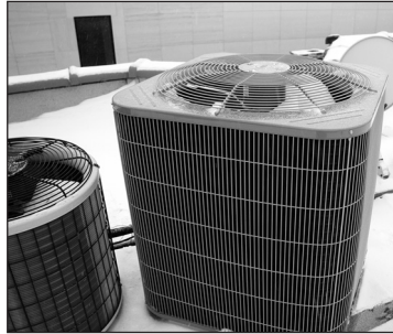
Air conditioning systems
