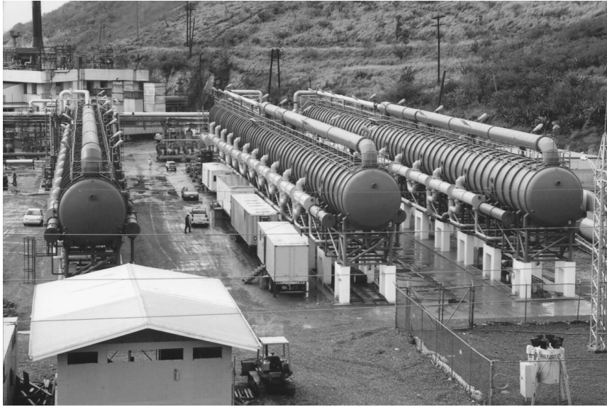
FIGURE 20.6.3 Two HTME desalination units, each producing 5000 m 3 /day, in St. Croix, U.S. Virgin Islands. (Courtesy of I.D.E. Technologies Ltd.)
