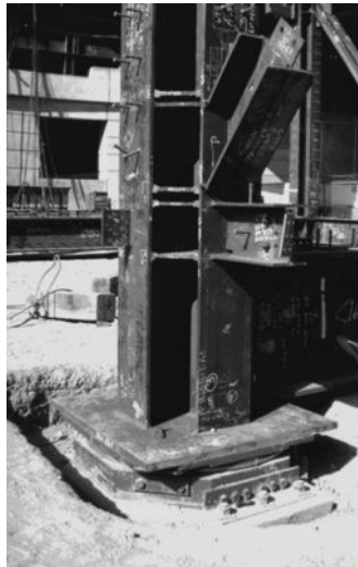
Figure 21.5.5 International Terminal at San Francisco Airport: FPS bearing at base of column. (P. Lee, photo, courtesy of Skidmore, Owings, & Merrill LLP.)
