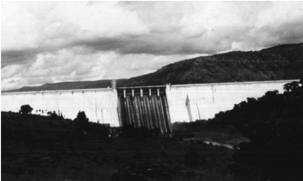
Figure 18.11.3 Koyna Dam, a 338-ft-high and 2800-ft-long concrete gravity dam near Poona, India. This major dam was damaged by the Koyna earthquake of December 11, 1967, a Magnitude 6.5 event centered 3 miles from the dam. [From A. K. Chopra, "Earthquake Response Analysis of Concrete Dams," in Advanced Dam Engineering for Design, Construction and Rehabilitation (ed. R. B. Jansen), Van Nostrand Reinhold, New York, 1988.]
