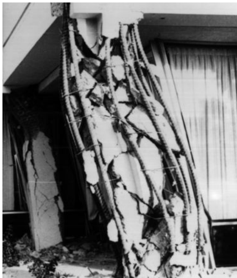
Figure 20.3.5 Brittle failure of a tied corner column of the Olive View Hospital building. (From K. V. Steinbrugge Collection, courtesy of the Earthquake Engineering Research Center, University of California at Berkeley.)
