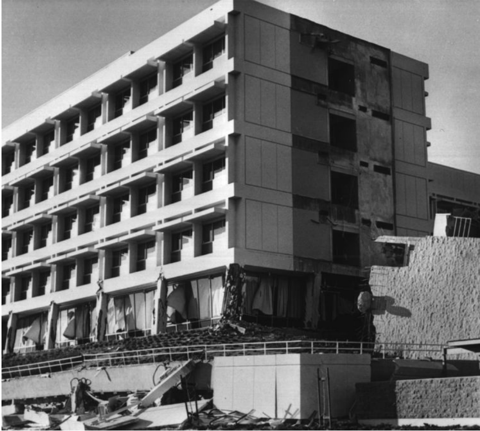
Figure 20.3.3 Olive View Hospital building. The shear walls in the upper four stories did not extend to the lower two stories. (From K. V. Steinbrugge Collection, courtesy of the Earthquake Engineering Research Center, University of California at Berkeley.)
