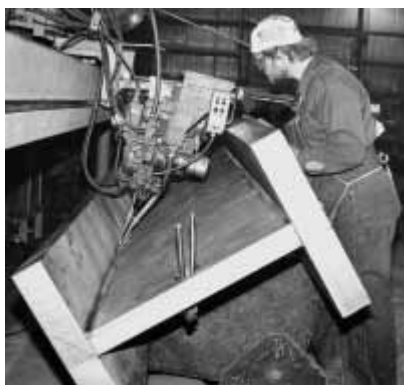
FIG. 5-17 Welding three large steel plates into a single solid section (Courtesy of The Lincoln Electric Company)
