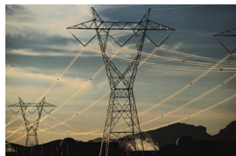
Photo 7.4 The forces on the supports and the internal forces in the cables of the power line shown are discussed in this section.
