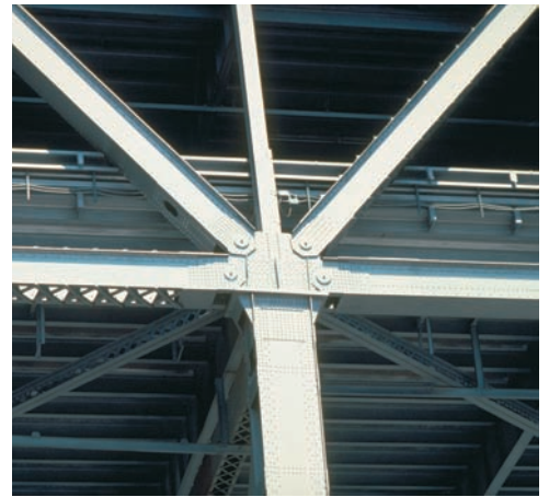
Photo 6.1 Shown is a pin-jointed connection on the approach span to the San Francisco–Oakland Bay Bridge.
