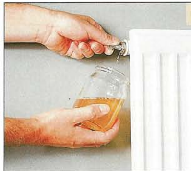
Dispensing an air pocket in a radiator
