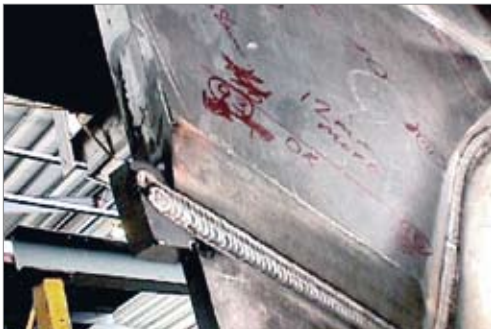
Figure 5. To match butt weld leg dimensions and facilitate even heat distribution heavier legs are tapered. Run-off tabs are used as appropriate.
