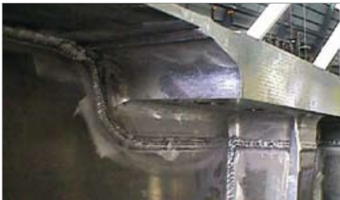
Figure 4. Weld designs for heavy sections include milling radii to relocate welds from fillet to butt positions.
