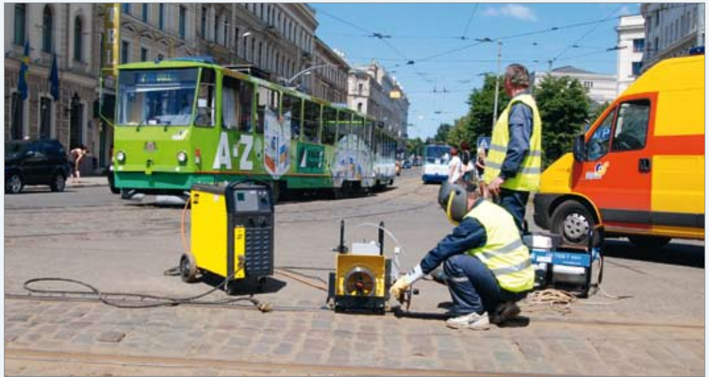
Figure 1. Small, lightweight and portable. Tramtrac™ II applied on tram rails in the streets of Riga together with the OrigoMig™ 410 power source.
