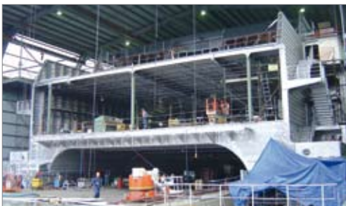
Figure 14. At the final assembly location "panamax" width hull 65 fully occupies Incat's 112m design shed height and width.
