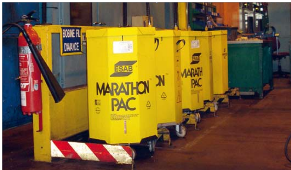
Figure 4. Four active Marathon Pacs, and a spare supplying a four-head installation for the welding of shock absorber housings.
