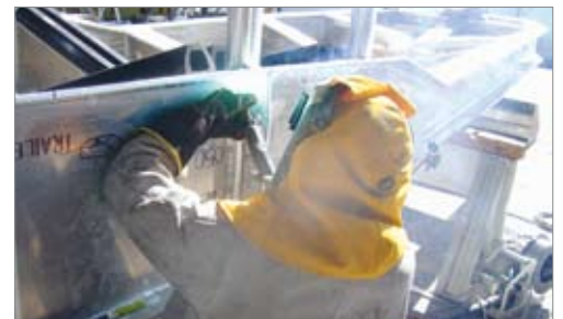
Figure 8. Uniform welding techniques, throughout the yard, produce uniform weld bead appearance and uniform weld quality.
