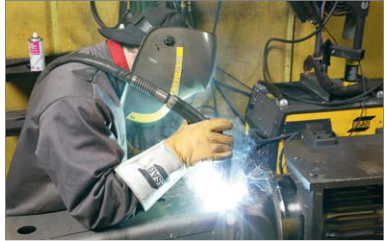
Figure 4. Manual welding of crucial safety components in the crane base with OK Tubrod 14.11-1.4mm. These welds need to have a full penetration and a perfect tie-in to provide high fatigue resistance. This joint is 100% US and X-Ray tested.
