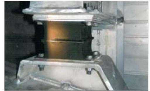
Figure 11. Rubber mounts isolate superstructure from sea frame.
