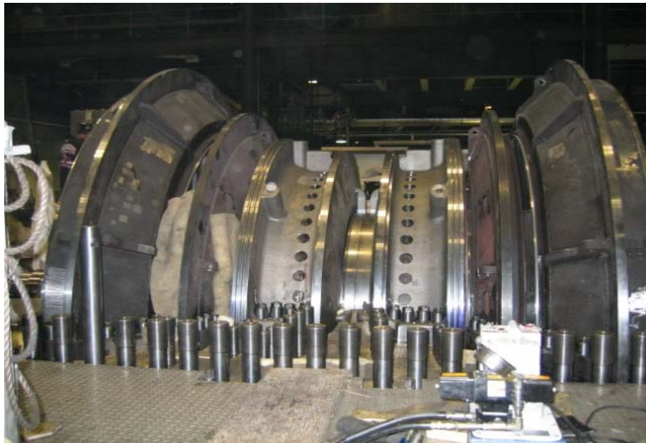
FIGURE 7 –LOW PRESSURE TURBINE REPLACEMENT FOR FOSSIL PLANTS
